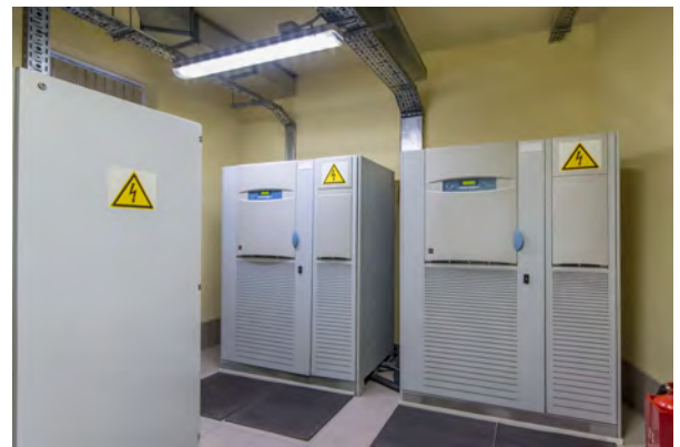
▲ Commercial/ factory UPS
